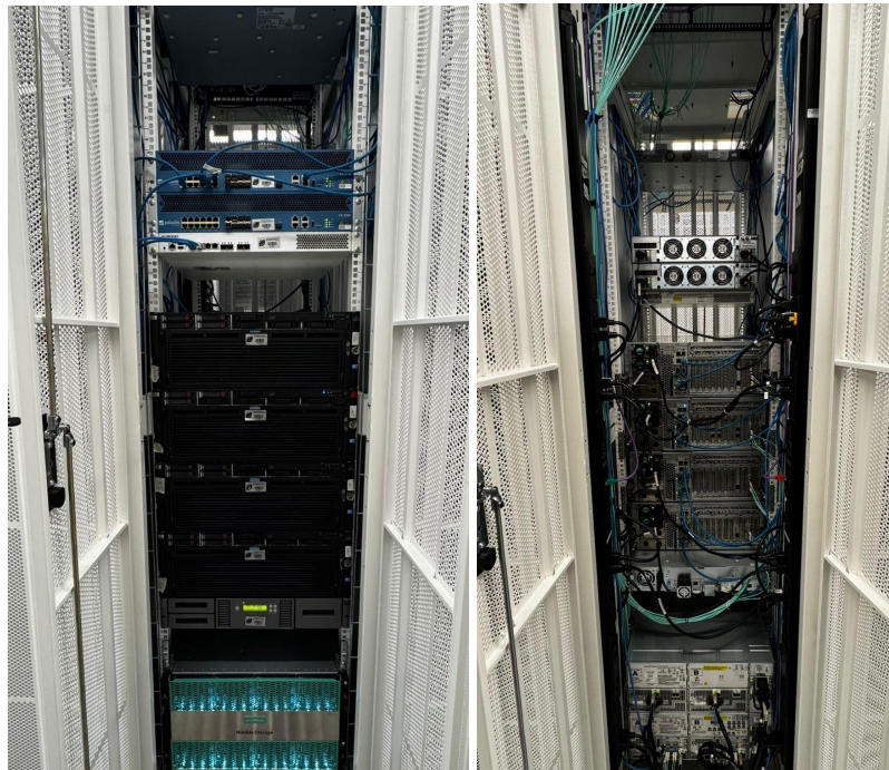
Figura 12 - Back & Front Rack 1G.12
