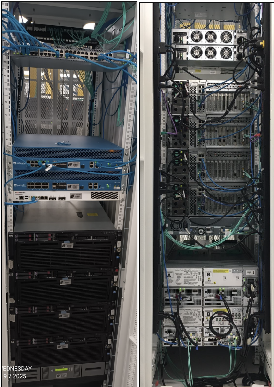
Figura 9 - Back & Front Rack 1G.12
