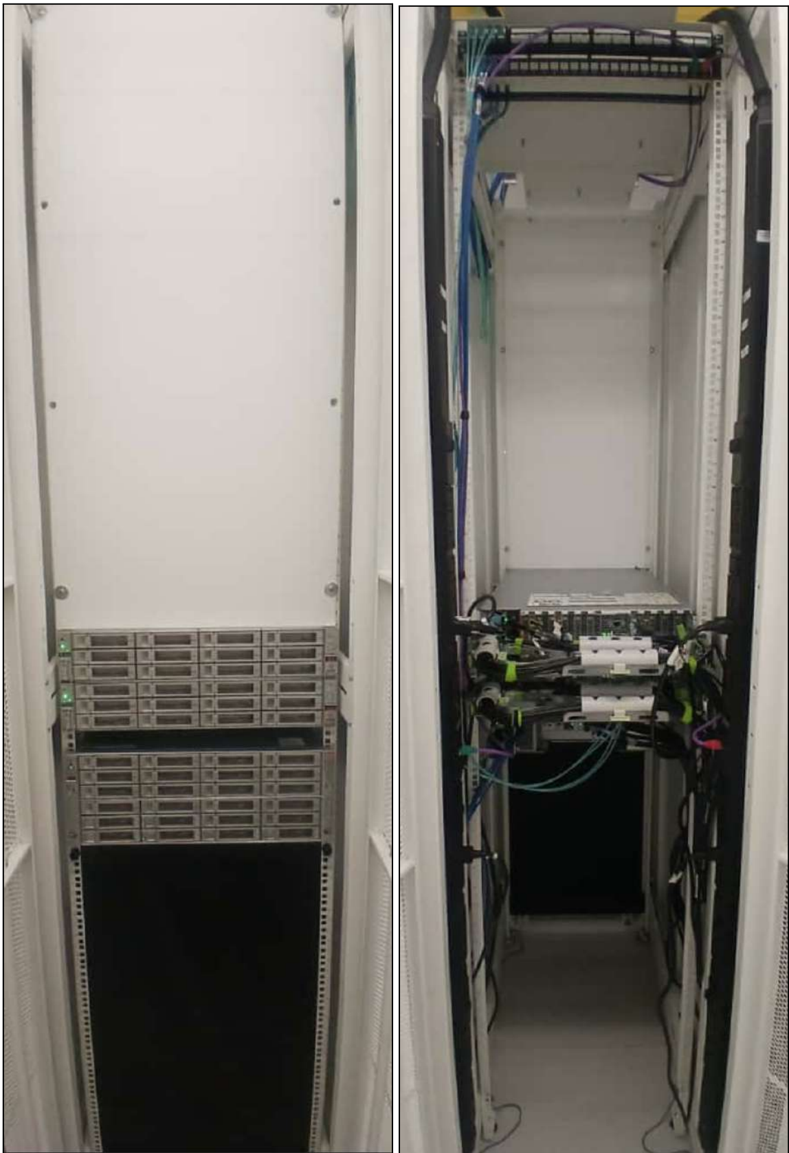
Figura 11 - Back & Front Rack 1H.11
