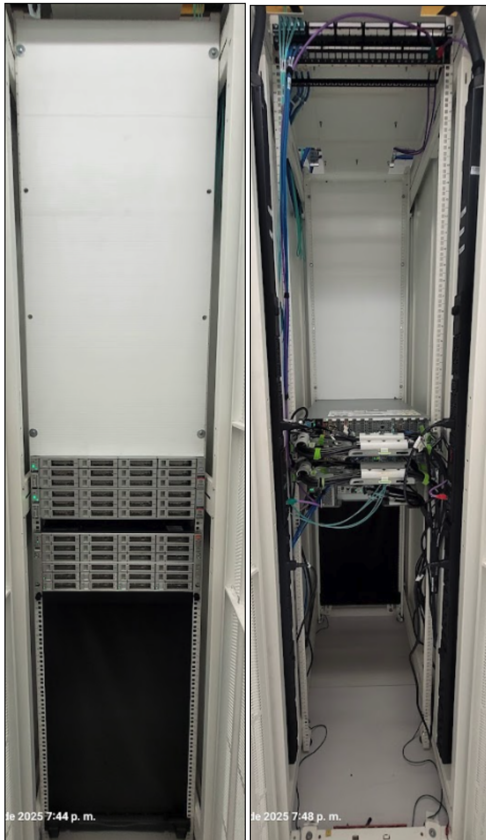
Figura 11 - Back & Front Rack 1H.11
