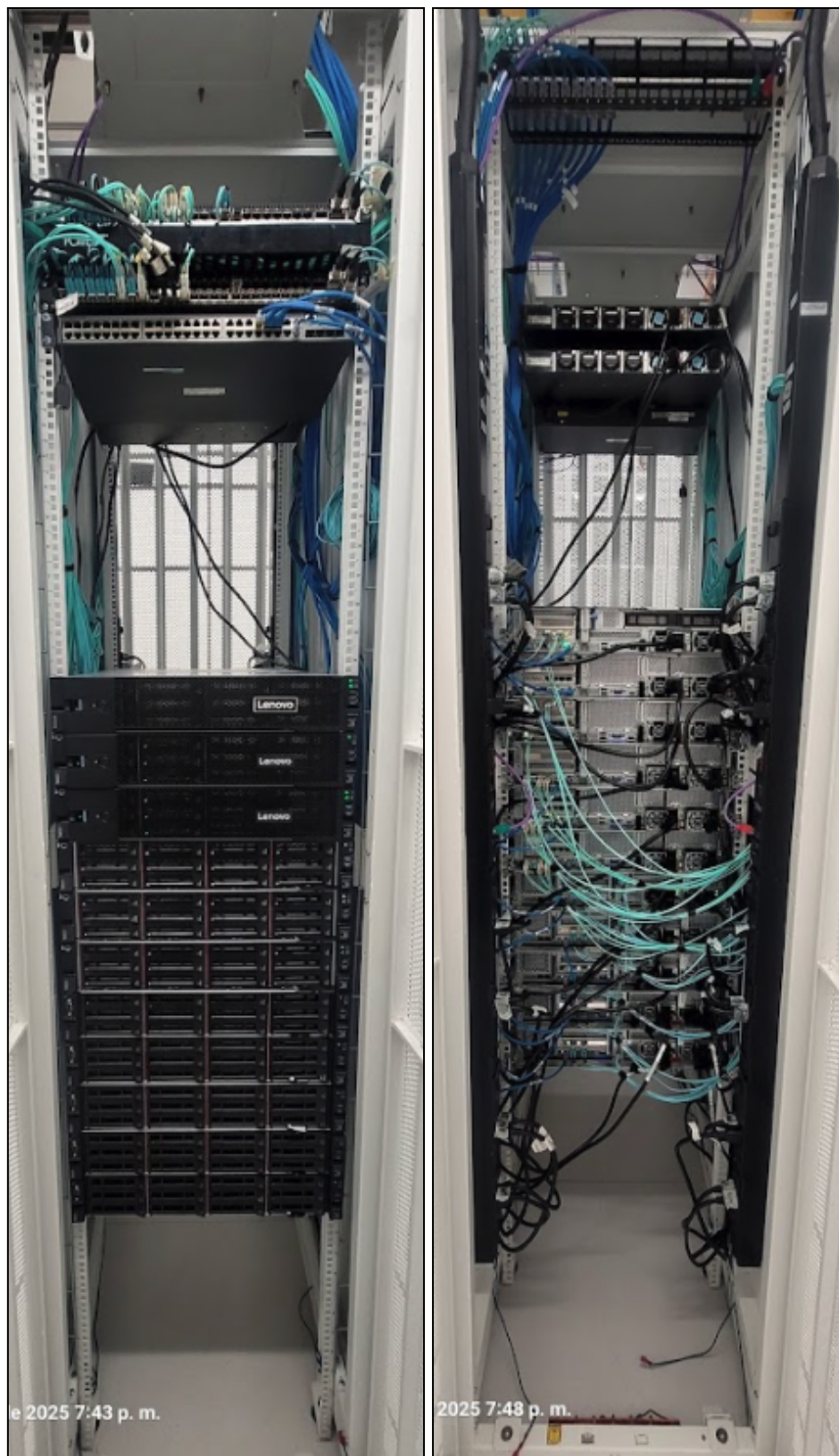
Figura 9 - Back & Front Rack 1H.09
