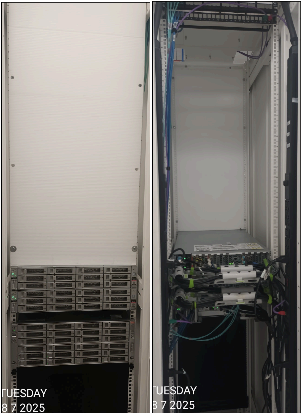
Figura 11 - Back & Front Rack 1H.11
